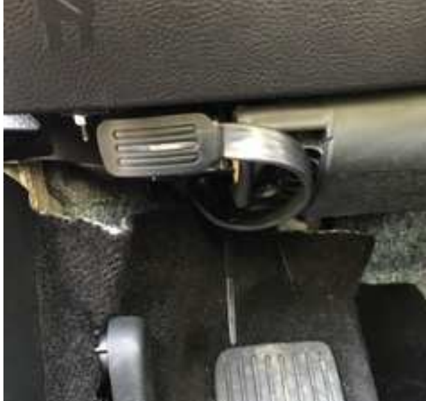
UTP 1.0 installed on 2017 Ford Fusion. UTP is routed and tie wrapped onto a wire harness behind the panel.
