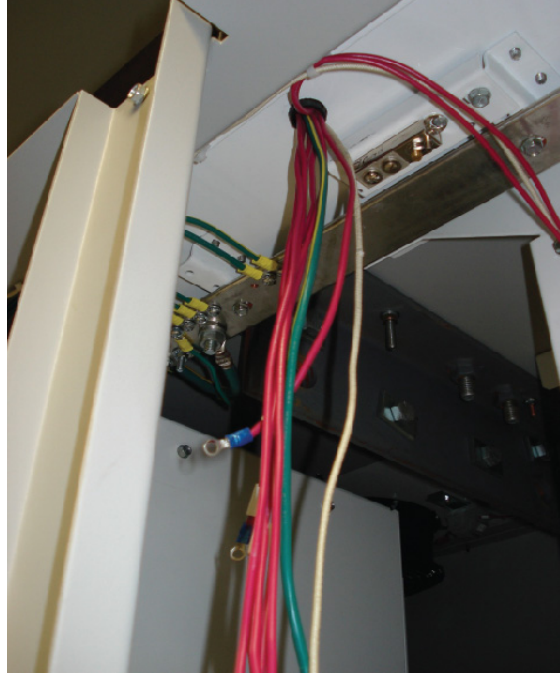
Figure 33 - Fan Thermostat Control Wires
