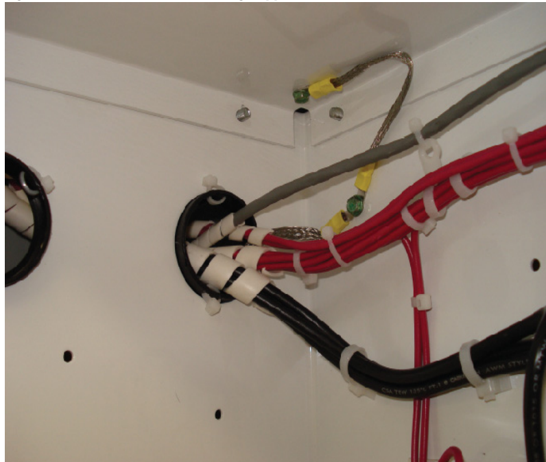
Figure 39 - 120V and XIO cables through upper cutout
