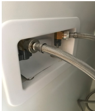
Water Shut-Off Valve
