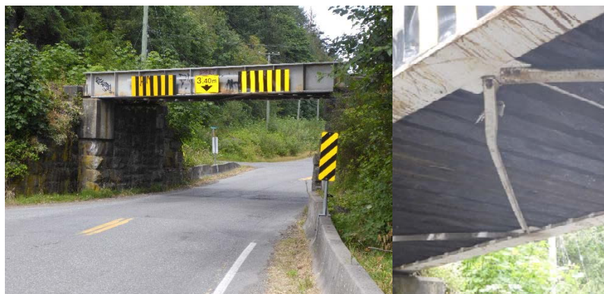
Figure 23: Shawnigan Lake Road Bridge Impact.
