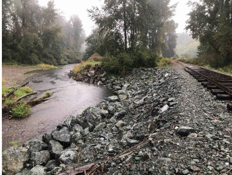
Figure 6: Washout at mile 37 – Victoria Subdivision
