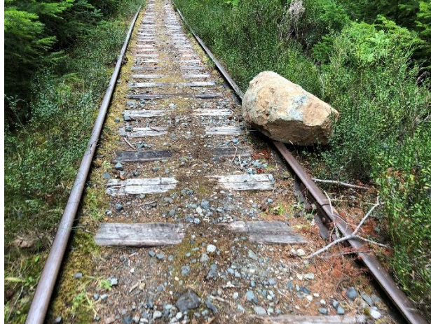
Figure 24: Rockfall Located on Port Alberni Subdivision
