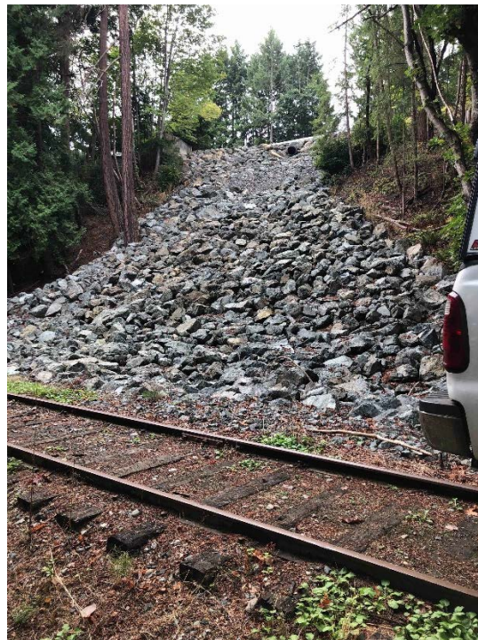
Figure 7: Washout at mile 84.4 - Victoria Subdivision
