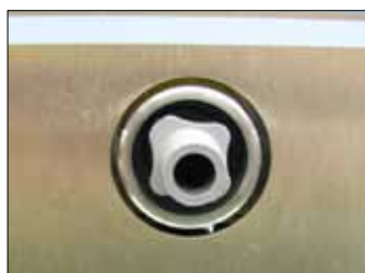
Installed Drain Fitting with Cap Removed
