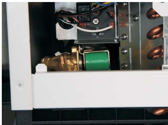
Inlet Water Solenoid Valve
