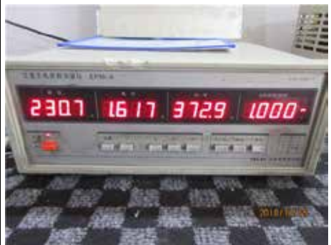
Power check at switch "fan II" and "Heat I"
