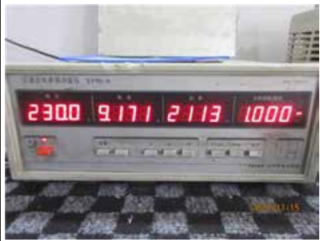
Power check at switch "fan II" and "Heat III"
