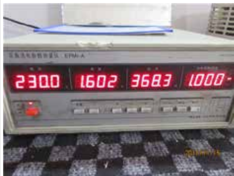
Power check at switch "fan II" and "Cool"
