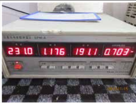
Power check at switch "fan I" and "Cool"
