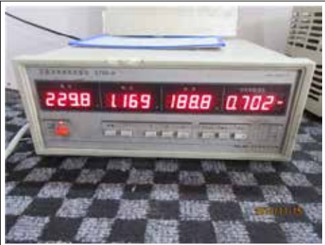
Power check at switch "fan I" and "Heat I"
