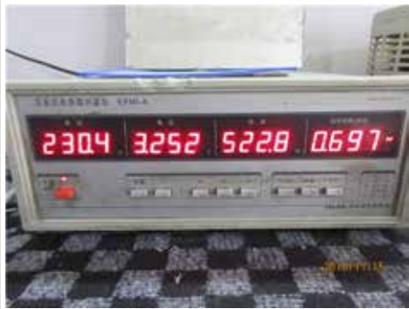
Power check at switch "fan I" and "Heat II"
