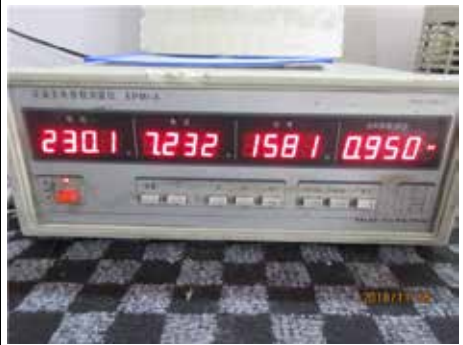
Power check at switch "fan I" and "Heat III"
