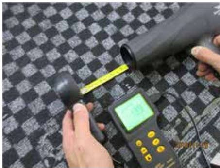
Air flow speed check
