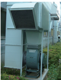
Exhaust vent with a noise reduction cover
