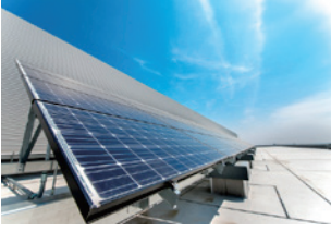
Solar power generators at the global headquarters building
