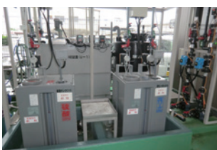
Neutralization segment of the industrial wastewater treatment facility
