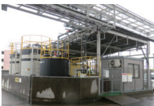
The industrial wastewater treatment facility
