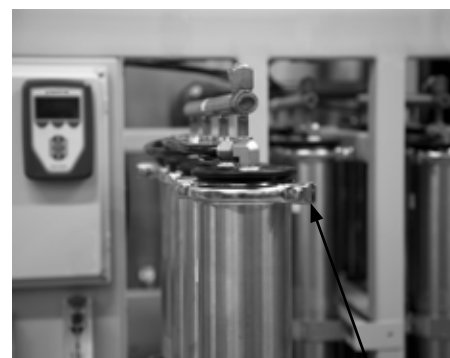
FIGURE 81-1: DRISTEEM REVERSE OSMOSIS MEMBRANES
