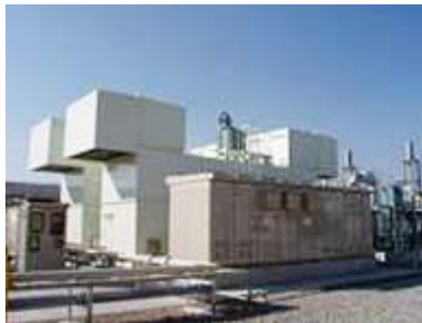
Cogeneration system facility
