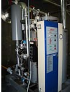
The natural gas-powered boiler at YMPI
