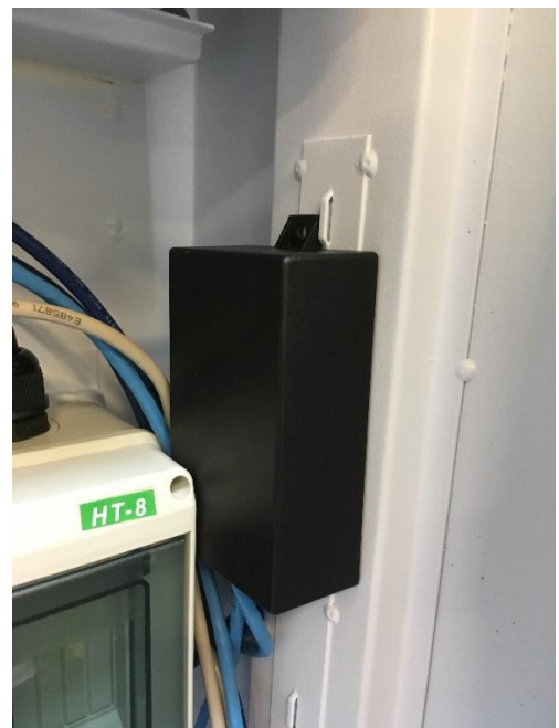
Fig 9: Black box placed adjacent to switch box
