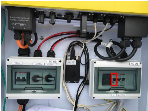
Fig 17: EMU power supply MCB
