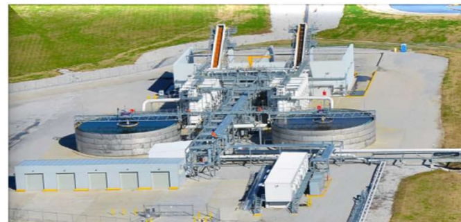
TVA has completed wet to dry CCR conversion at 4 out of 5 operating coal plants
