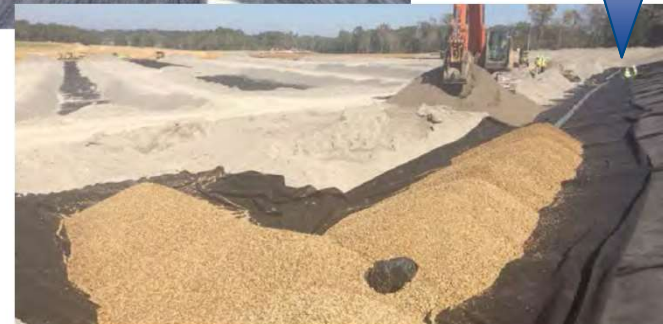
Leachate Collection Pipe
