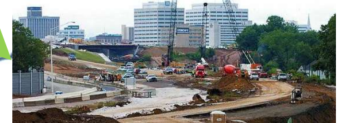
TDOT Smartfix Project Utilized Bull Run and Kingston Fly Ash in concrete mix designs
