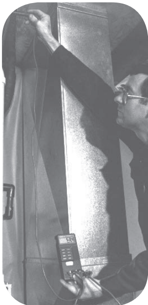
FIGURE 48 TEMPERATURE RISE MEASUREMENT
