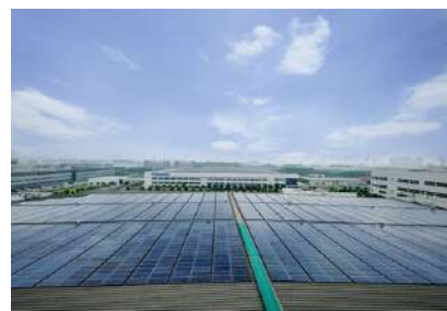
Photovoltaic power generation system in PAPCN
