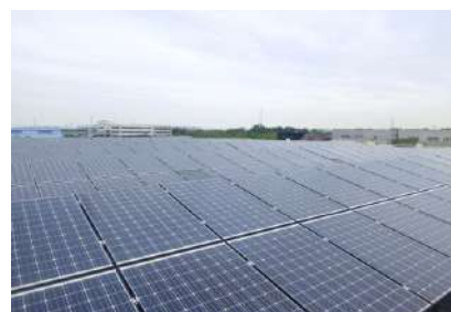
Photovoltaic power generation system in PMFBJ
