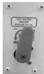
Water Heater Bypass
