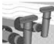
Low Point Drains
