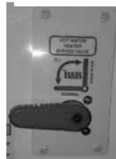
Water Heater Bypass
