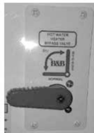
Water Heater Bypass
