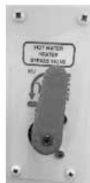
Water Heater Bypass
