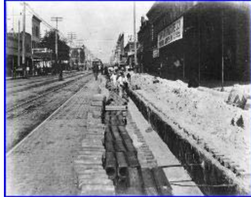
1903 Road construction on Florida Avenue in front of the Tampa Furniture Company (707-709 Florida Avenue) in Hillsborough, Fla. Seen are a crew of construction works in a water main ditch, mixed brick and stone paving, and the street railroad tracks. A black and white photograph in jpeg format contributed by: Burgert Brothers. Tampa System number B29-00042357
