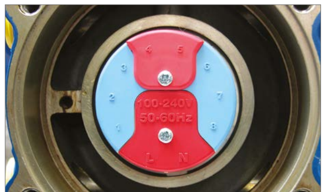
Fig 7.16 IS Terminal Block
