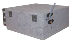
Metal parts insulated to avoid condensation
