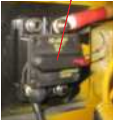
Located on battery box
