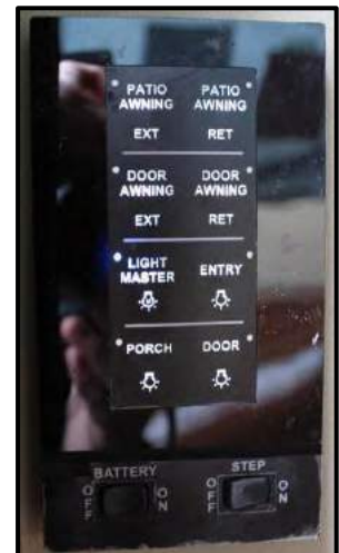
Figure 9-16: 12 VDC Disconnect Switch
