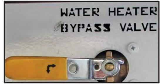
Figure 13-9: Water Heater Bypass System
