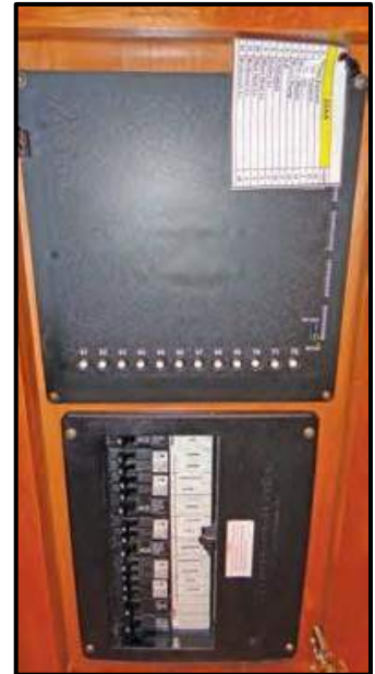
Figure 9-3: Circuit Breaker Boxes
