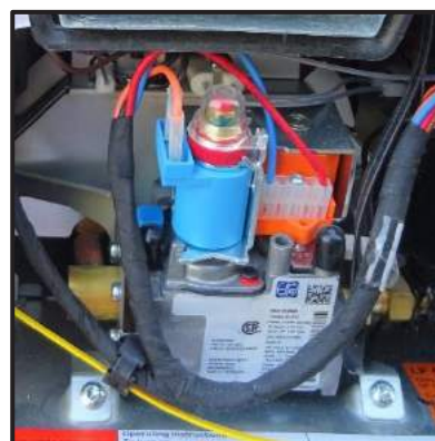
Figure 5-10: Water Heater Relief Valve
