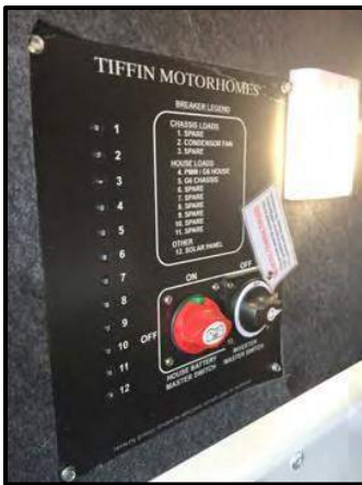
Figure 9-14: House Battery Disconnect Panel
