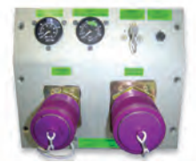
Ground Service Panel
