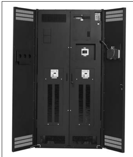
Figure 1.1-18. Power Distribution Unit
