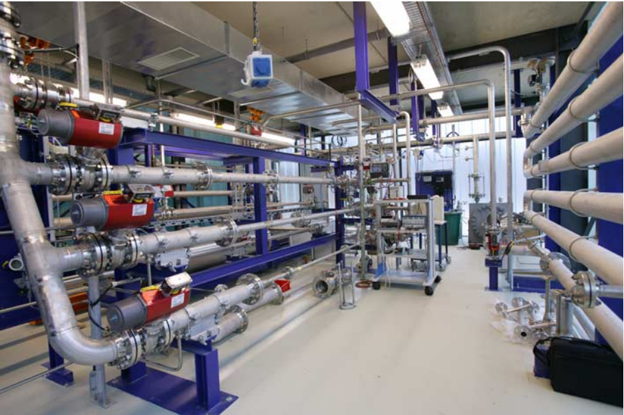
Fig. 3-21: Pictures of the Process Gas System
