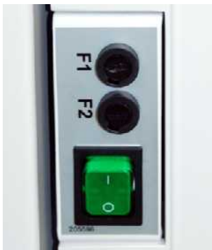
Fig 1.1. On/off switch and main fuses
