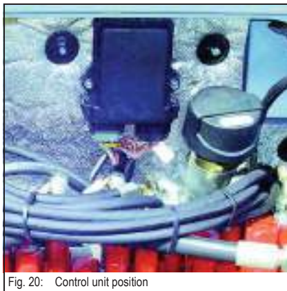
Fig. 20: Control unit position
