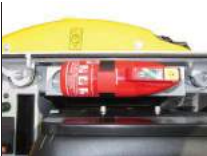
Fig. 92: Fire extinguisher in canopy
