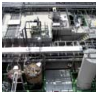
Wastewater treatment system
