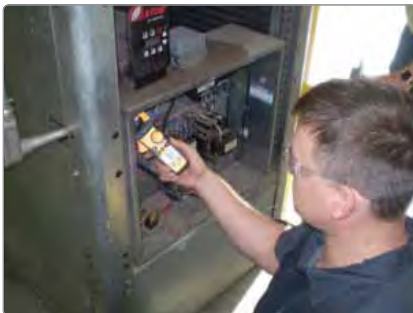
Cummins employee Mike Garrett looks for potential energy savings as part of the Company's Energy Champions program. The low and no-cost improvements uncovered by Energy Champions and Leaders are critical to energy efficiency efforts going forward.
