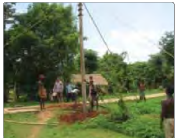
Village residents help with the installation of the poles and wires necessary to bring power from the Cummins' generator to individual homes.
