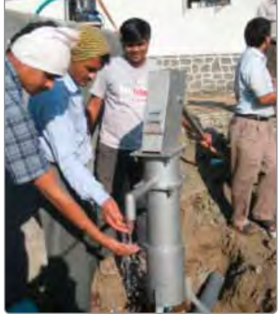
The team on the Wagholi project installs a hand pump to help teach students that pumping water is hard work and that water should not be wasted.
