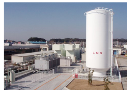
Cogeneration equipment at Kakegawa Factory
