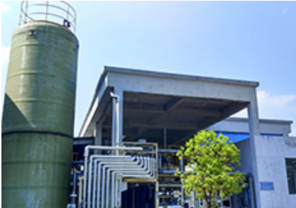
Wastewater treatment facility (Xiaoshan Yamaha Musical Instrument Co., Ltd.)
