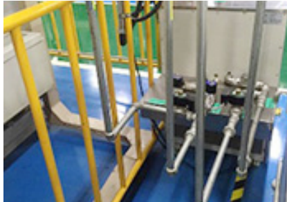
Cooling unit using circulated water (Xiaoshan Yamaha Musical Instrument Co., Ltd.)
