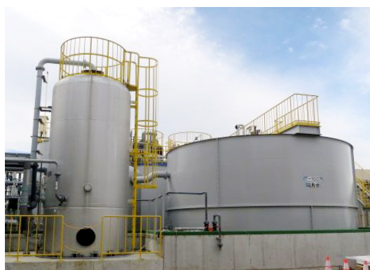
Wastewater processing equipment at the headquarters factory of Yamaha Music Manufacturing Japan
