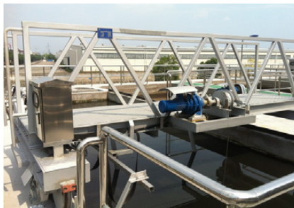
Reusing wastewater for cooling water (Hangzhou Yamaha)
