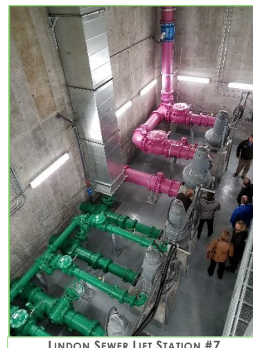
LINDON SEWER LIFT STATION #7
