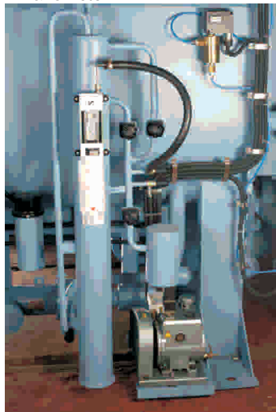
The Purge System
