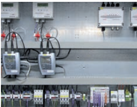
Measurement equipment in switch cabinet.
