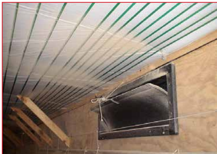
Figure 36: Example of a good quality air inlet.
