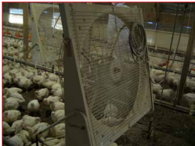
Figure 29: Circulation fans in a naturally ventilated house.
