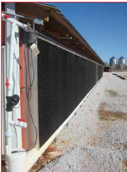
Figure 45: Example of a cooling pad installed on the sidewall of the house (in a 'doghouse').
