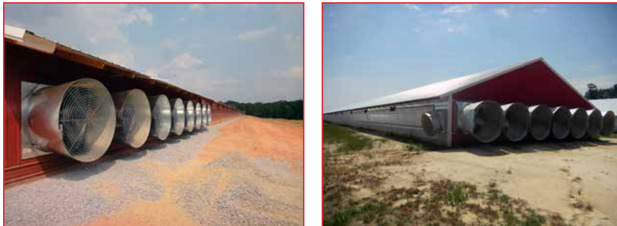
Figure 40: Example of a typical tunnel ventilated house.
