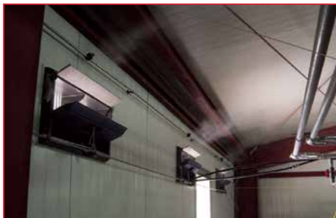
Figure 46: Example fogging system for a cross ventilated house.
