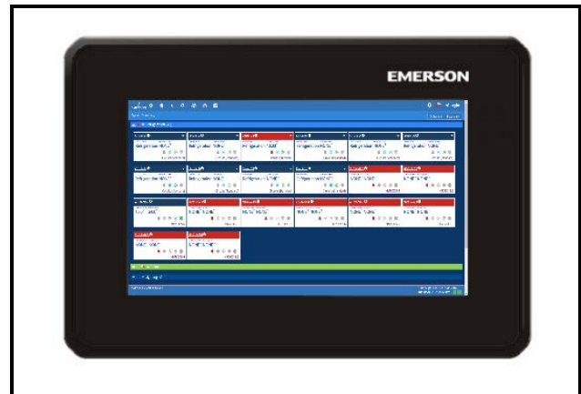
Figure 5-18 - Supervisory Controller Display
