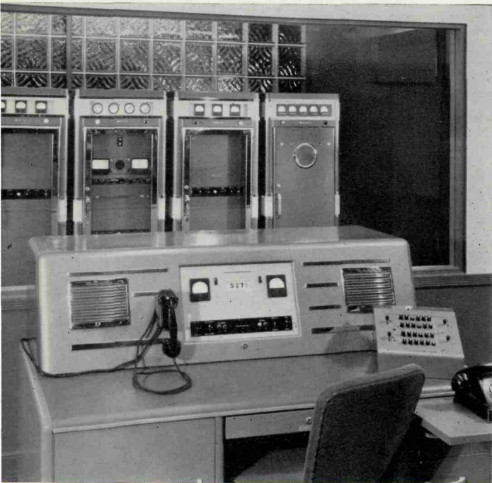
Recent Installation of Motorola Two-way FM Communication System for Both a Community Police and Fire Department
