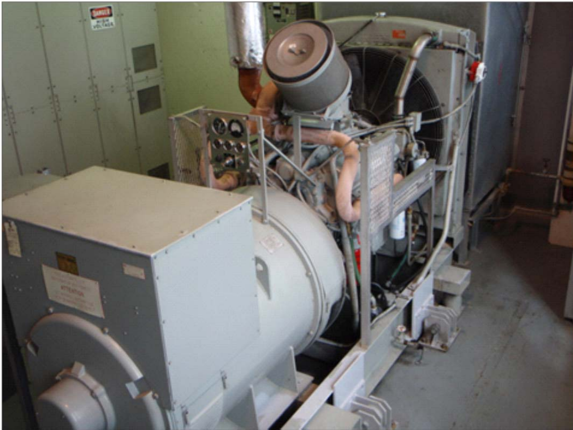
Figure 3-7. Diesel-electric generator set (source: Toronto International Airport)
