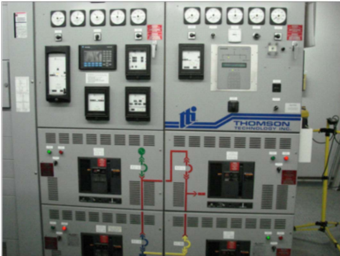
Figure 3-8. Transfer panel (source: Toronto International Airport)
