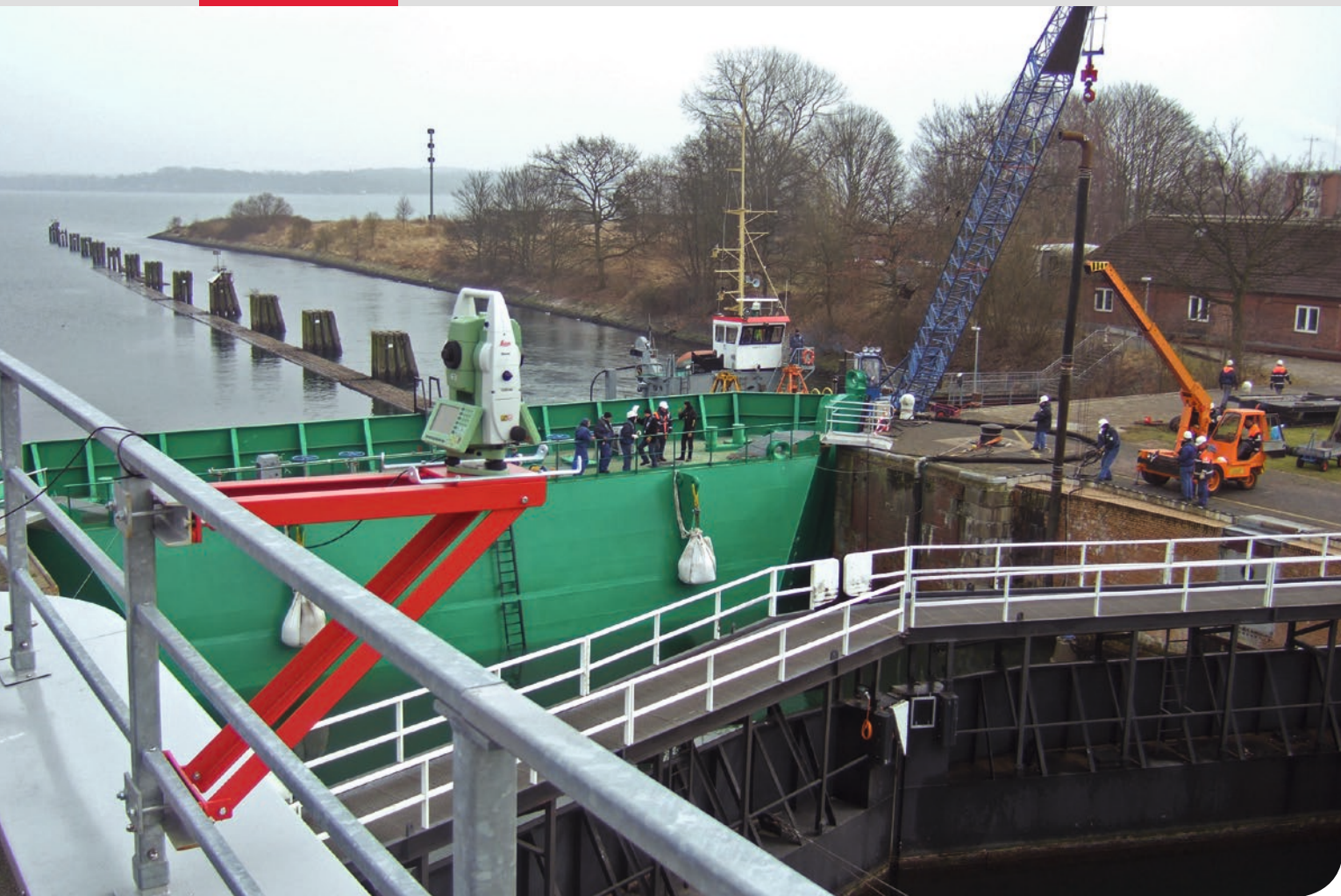
■ A Leica Geosystems total station takes measurements to observe possible movements of the chamber wall.
