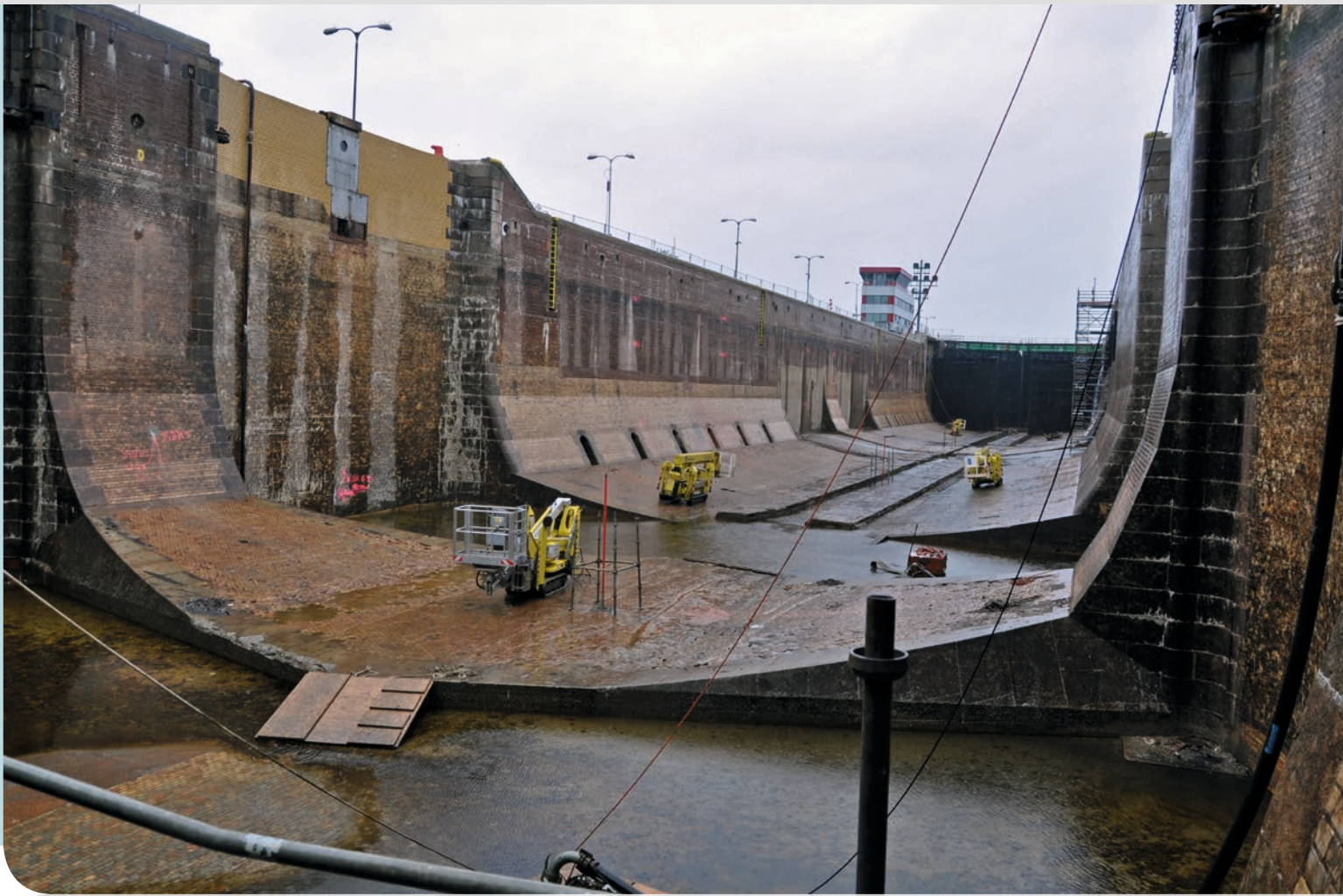
■ Ready for safe renovation: The empty ship lock gets inspected while the structure is being monitored.
