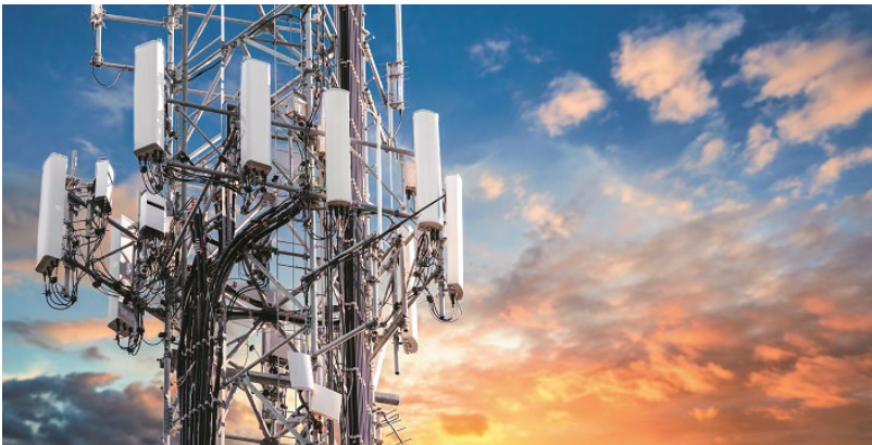
Figure 8: Antenna pointing systems – base and rover on single-cell antenna panel
