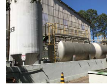
Rainwater storage facility (FUJIFILM do Brasil Ltda.)
