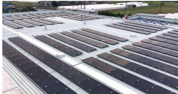
Photovoltaic power facility in FFTP Sano Site
