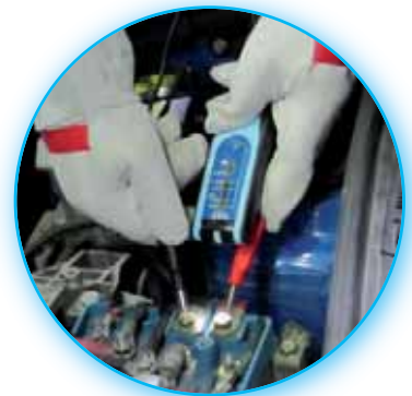
Voltage detection on electrical power circuit.
