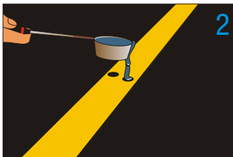
The holes are filled with bitumen
