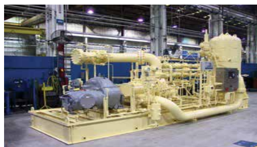
Steam turbine-driven driveline, Indonesia
