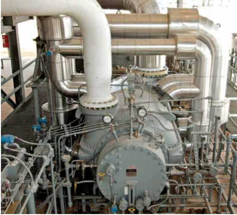
4,000-hp driveline in gas-processing application
