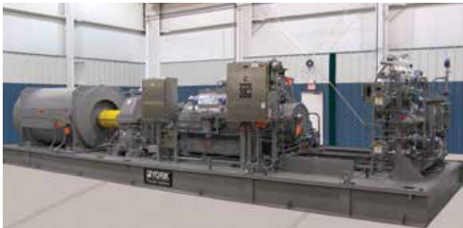
Distillation column heat pump, U.S.
