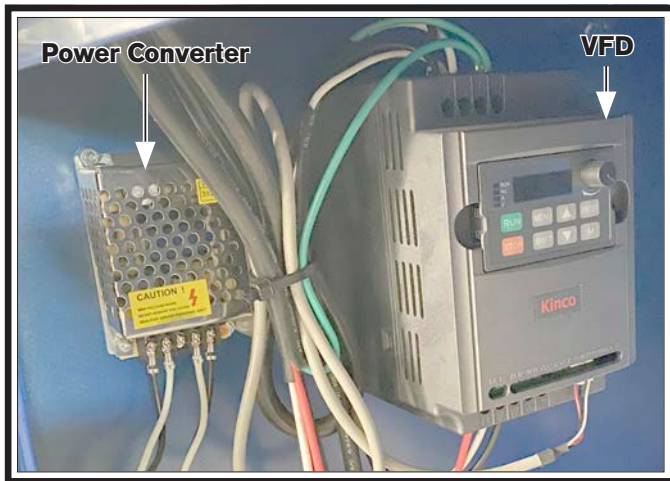
Figure 91. Electrical components inside cabinet.
