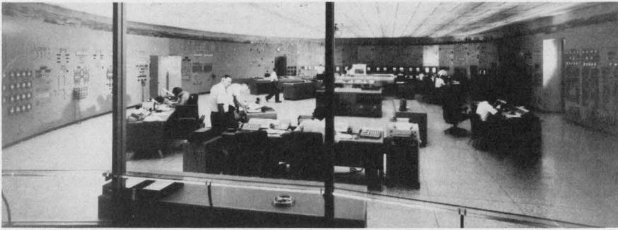
Technicians monitor and control power flow through 325 substations from Con Ed's Energy Control Center.
