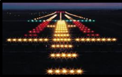
LED Runway Lighting and EFVS
