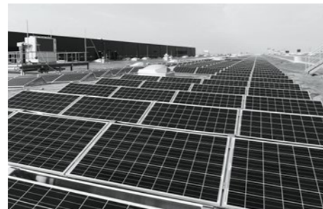
PHOTOVOLTAIC SYSTEMS AT LEIPZIG PLANT
