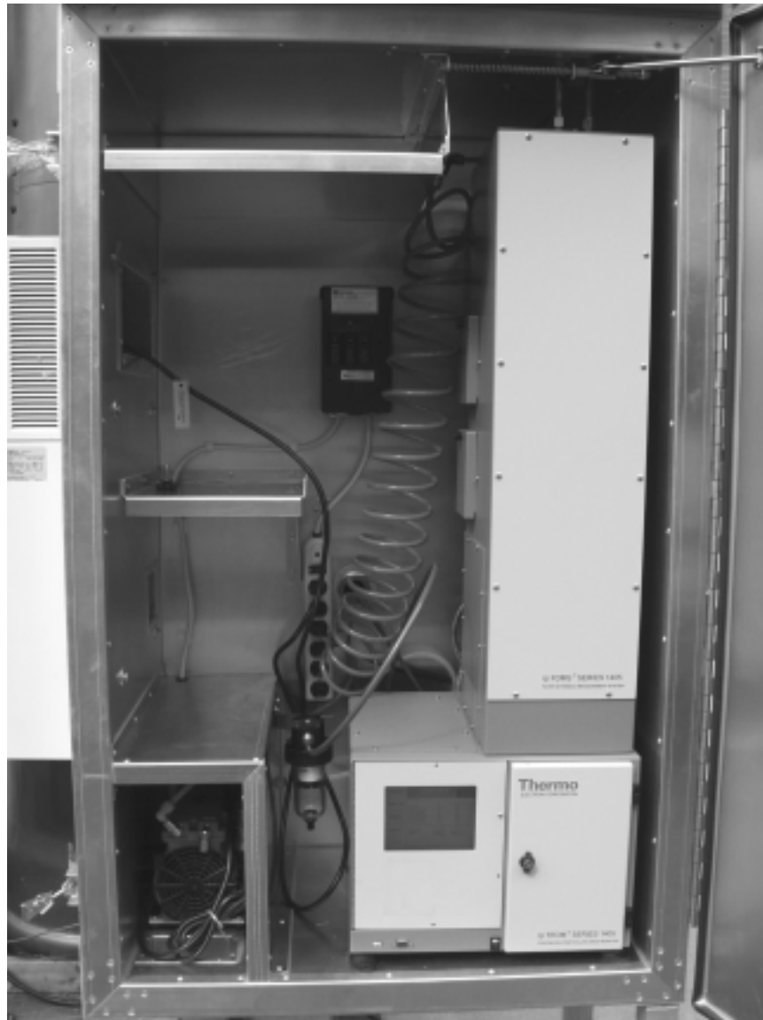
Figure 2-18. 1405 unit in the outdoor enclosure (FDMS unit pictured).
