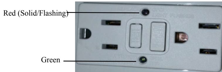
Figure 3. NEMA 5-15 Receptacle Lights
