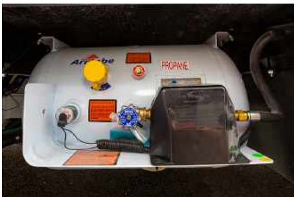
Figure 39.1 LP Propane Gas Tank
