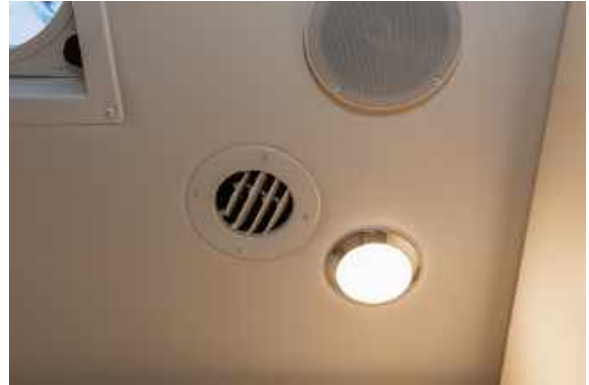
Figure 35.2 Roof Mounted Round Air Vent with Directional Air Guides Opened
