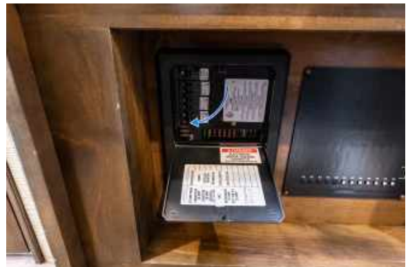
Figure 73.2 Wayfarer Breaker Box Located with 30AMP Main Breaker Highlighted by Blue Arrow
