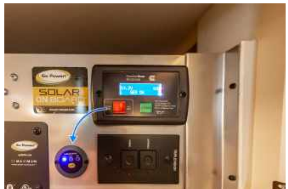
Figure 81.2 Inverter Switch Located on Central Control Panel Usually in Bedroom Area of Motorhome
