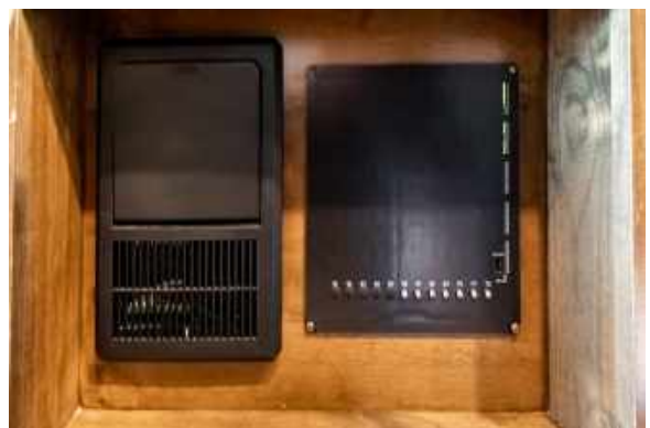
Figure 75.2 Wayfarer 12VDC Box Located Next to 12VAC Circuit Breaker Box in Bedroom Area of Motorhome
