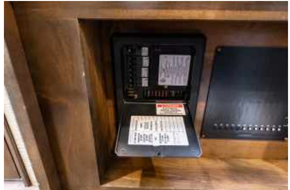
Figure 75.1 Wayfarer 120VAC Breaker and Fuses Located in Bedroom Area of Motorhome
