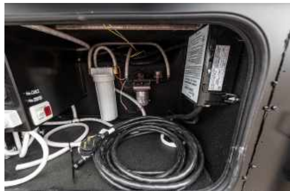
Figure 72.2 Wayfarer 30AMP Power Cord in Exterior Compartment
