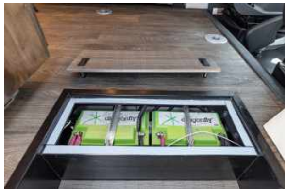
Figure 77.2 Access Panel Removed Exposing Coach Batteries *Optional Lithium Batteries Shown
