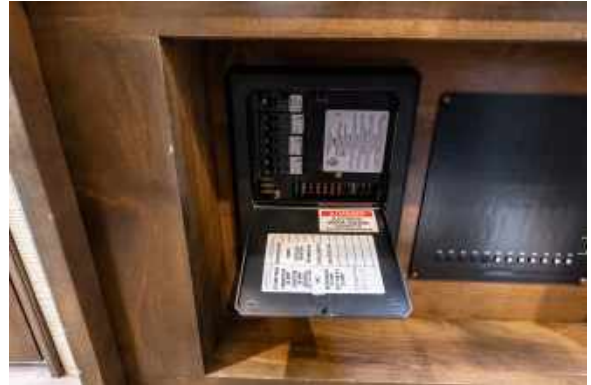
(Figure 84.1) Circuit Breaker Box Located in Bedroom Area of Motorhome
