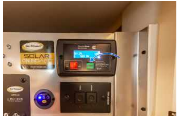
Figure 82.2 Remote Generator Start Switch Located on Central Control Panel
