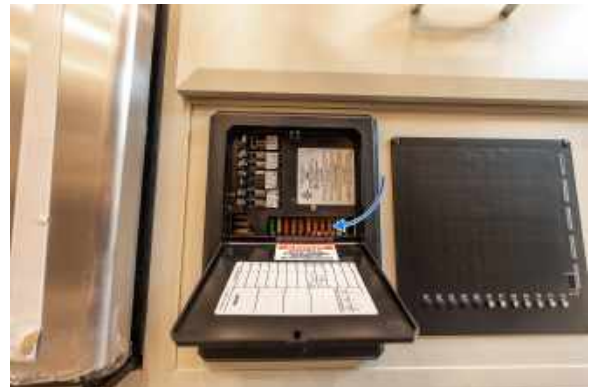
Image 64.1 Fuse That Controls the Power to the Tri-Fold Sofa Power System
