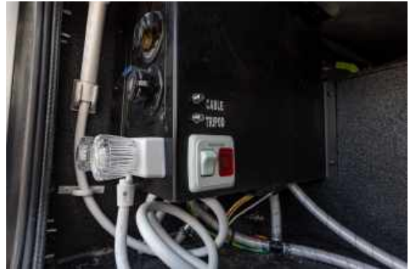
Figure 54.2 Wayfarer Exterior Satellite/Cable Input. Located in Driver's Side Rear Most Exterior Compartment.
