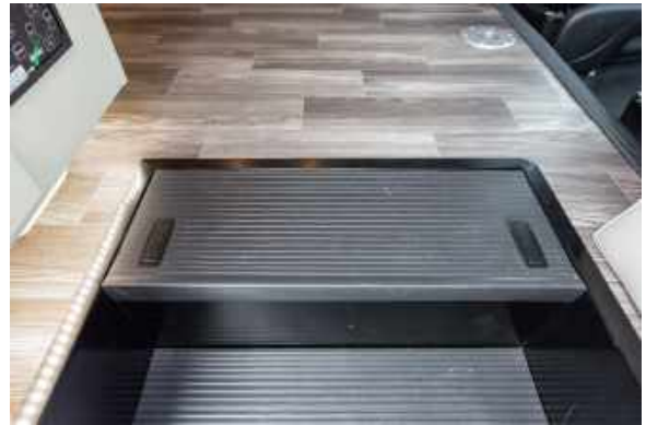
Figure 77.1 Coach Battery Located Inside Entry Step Well
