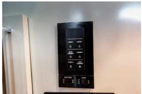
Figure 97.2 Security/Patio Light Control on Panel Just Inside Rear Entry Door to Motorhome
