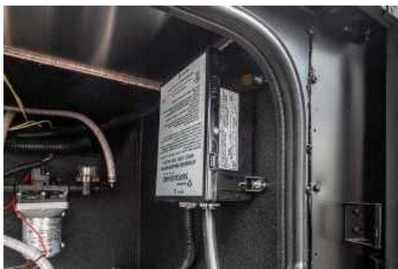
Figure 83.1 Automatic Transfer Switch
