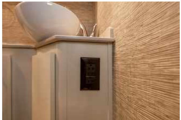
Figure 80.2 GFCI Receptacle Located in Bathroom Area
