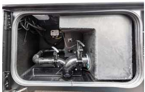
Figure 114.1 Sanitation Coupling with Gray and Black Water Tank Gate Valves
