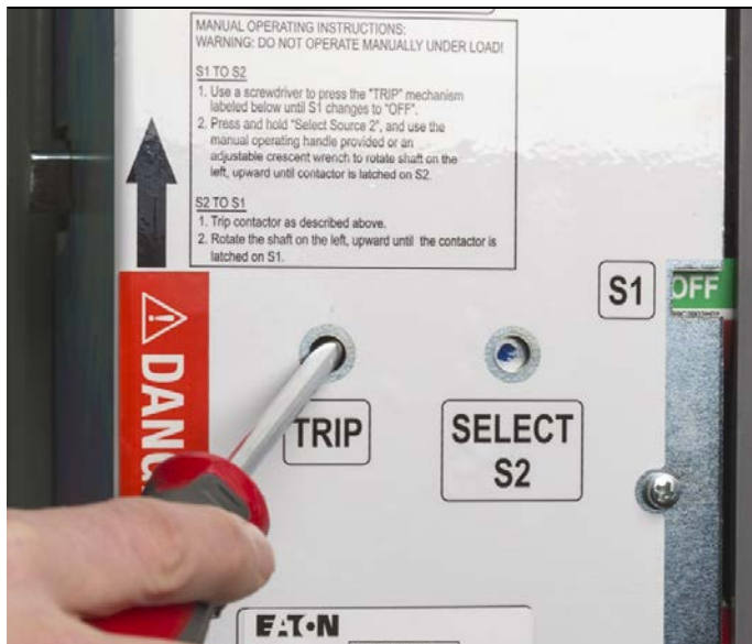
Figure 12. Trip Button on Contactor Operating Mechanism.
